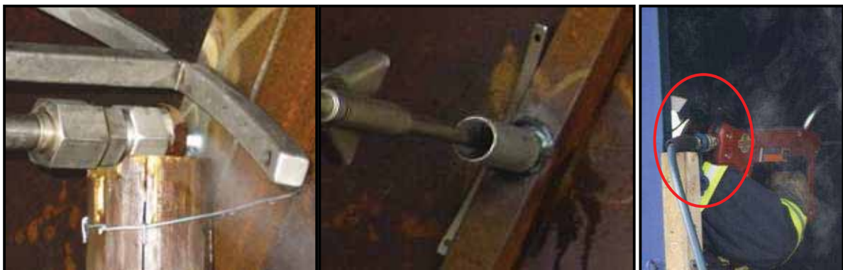
Figure 28. Left & middle: First guide, later replaced by a steel cylinder / Right: Wedge used to preserve perpendicularity with the pierced wall [and then being exactly parallel with floor and vertical walls]. Picture: Service Communication SDIS68
